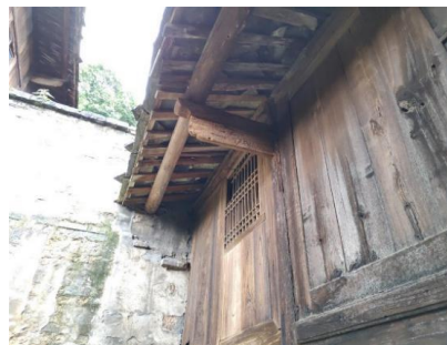
Figure2-1-3 The stigma purlin bearing method of traditional buildings in Benzhai Source: Author's own photos
