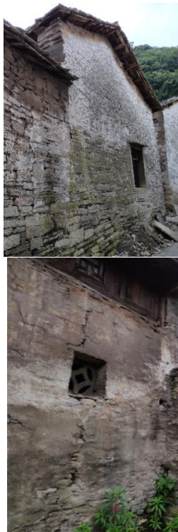
Figure 2-2-1 Breakage of wall Source: Author's own photos
