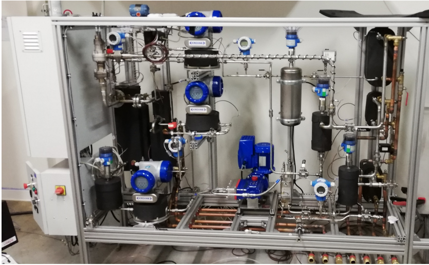
Figure 1. Picture of the pilot plant.
