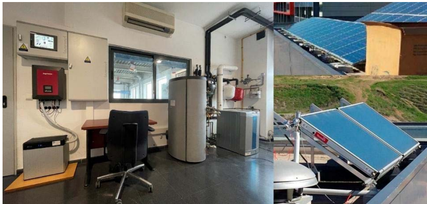
Fig. 1. Image of facilities. (On the rooftop and inside the laboratory).
