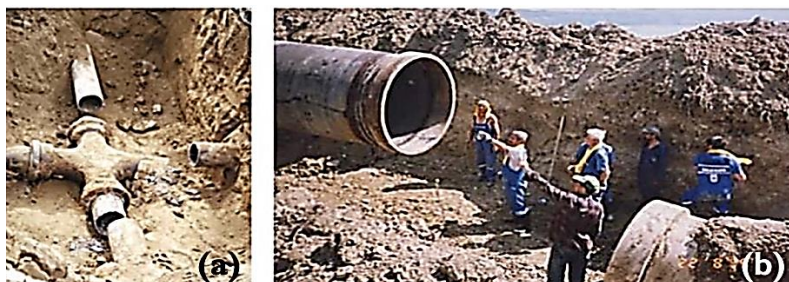
Figure 4. Failure pipelines modes because of mechanical joint root out in the (a) 2011 Christchurch seismic; as well as (b) Tohoku 2011 [23].
