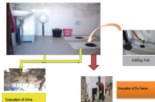
Fig. 2. UDDT installed at Dayet Ifrah Village
