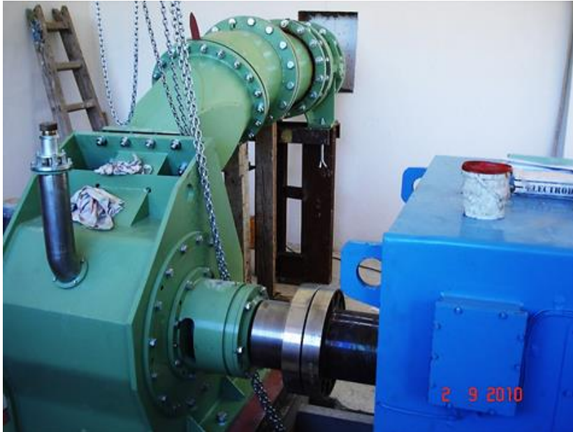
Fig. 8. Hydropower unit (Tufcha 1 HPP).
