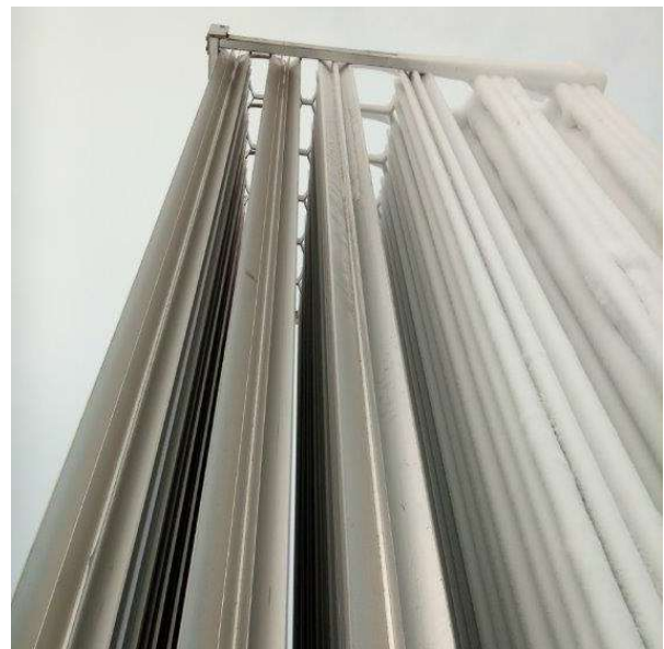
Fig. 1. Longitudinal finned tubes with accumulated ice.
