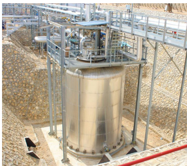
Fig. 4. Underground molten salt TES system (14 MWh thermal) integrated with super-heated steam generator developed in the project MATS [6].
