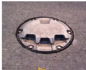
Fig.1. An embedded airport navigation lamp.
