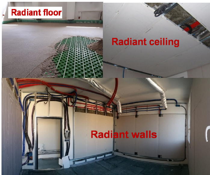
Fig. 2. Radiant systems installed in CORE-CARE laboratory.
