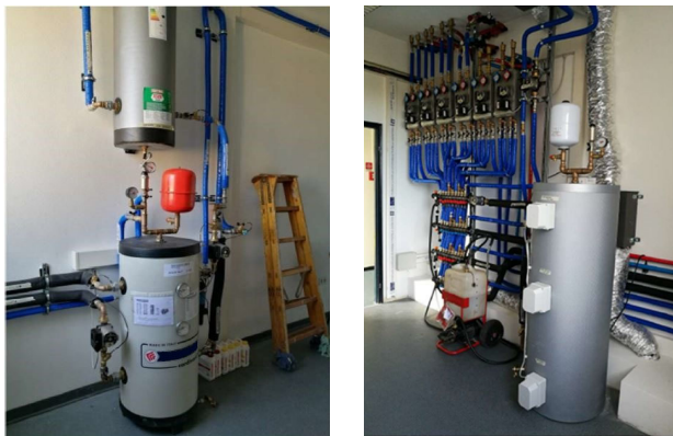
Fig. 3. Cooling tank and connection with chiller circuit (left); heating tank and secondary circuits (right).
