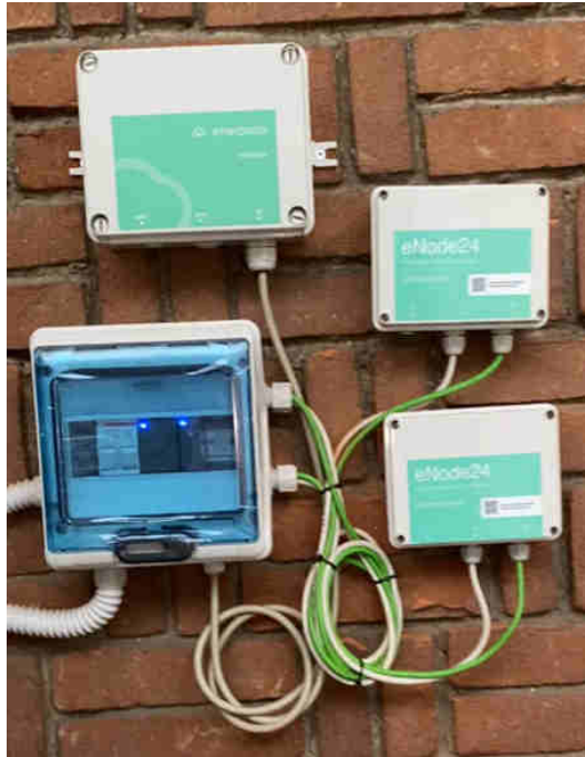
Figure 1. IoT controllers controlling the fan and the pre/post-heating valve of Nuclear Medicine AHU.
