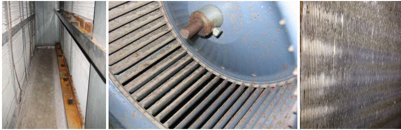
Fig.6 – Evident state of degradation with the generation of products, from oxidation and corrosion of metals and / or insulation materials, which combined with condensed water or humid air can in turn give rise to chemical substances that can be harmful to inhalation by people
