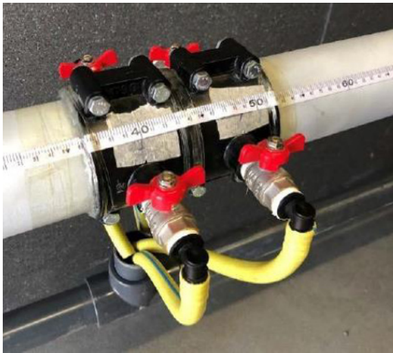
Fig. 3. Artificial leakages by means of valves and plastic tube that used to avoid any flooding inside the container
