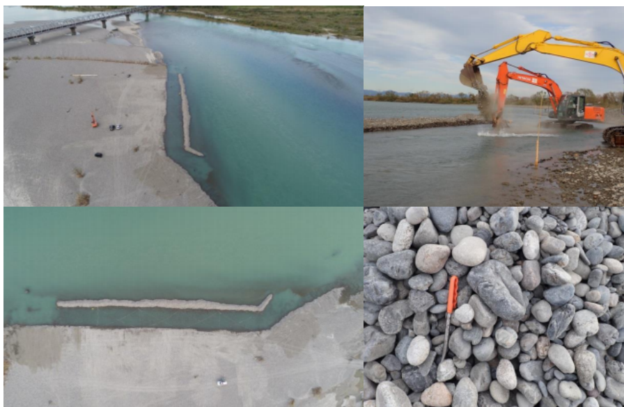
Fig. 9. Diagonal and vertical aerial shots taken immediately after the completion of construction on November 1, 2018 (top and lower left); Throwing of gravel and gravel thrown in the channel (top and lower right).
