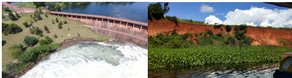
Fig. 4. Excessive erosion and slope collapses.
