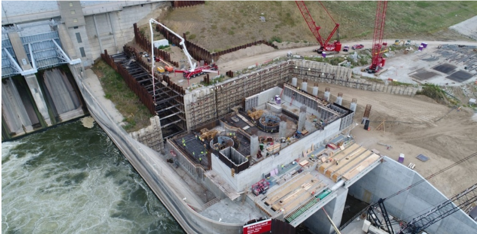
Fig. 5. Aerial photograph of the downstream penstock, powerhouse, and tailrace features (photo provided by MRES).
