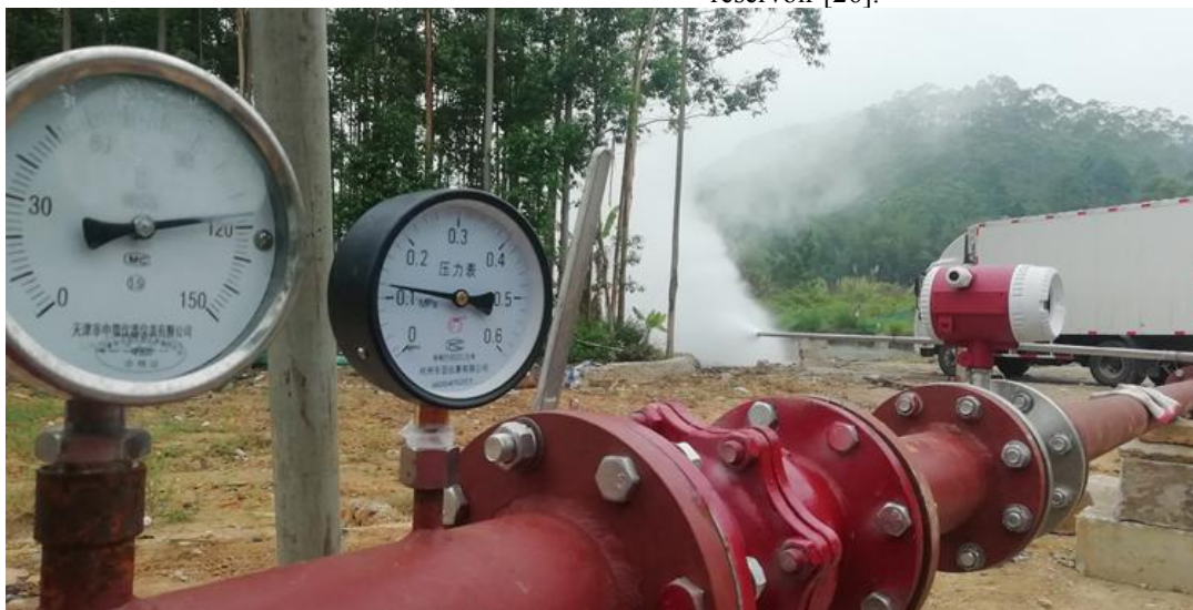
Fig. 3. Data collection system of thermal storage test of Well Huire-1
