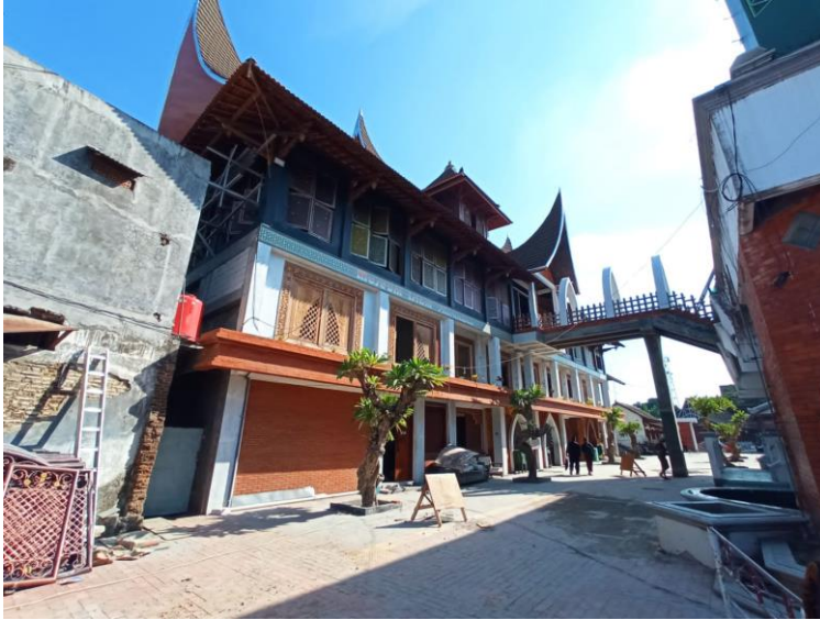
Fig. 2. The building of The Islam Nusantara Museum which stores ancient manuscripts that are damaged and not well preserved
