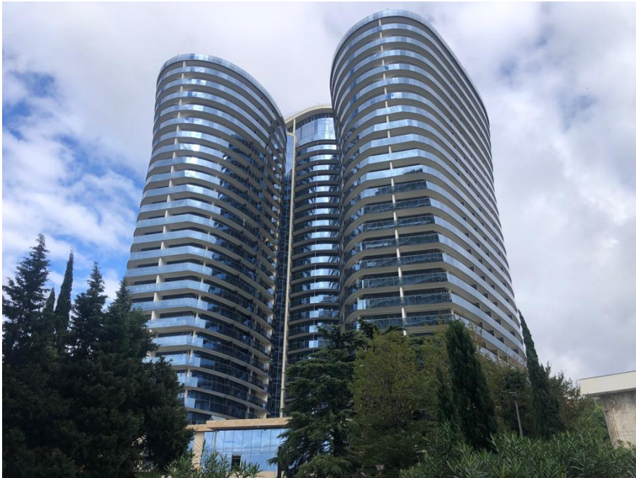
Fig. 7. High-rise building of complex shape on Kurortny Avenue in Sochi: the final stage of the construction of the facility.
