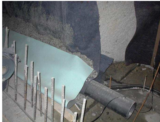
Fig 4. Drainage pipe installed at the base of the spring, surrounded by the drainage layer and the barrier layer, i.e. geomembrane
