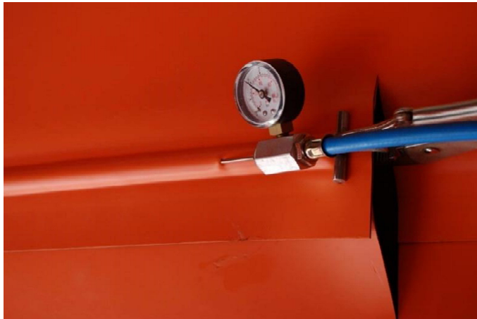
Fig 6. Geomembrane welding control with pressured air in the channel between the double welding.
