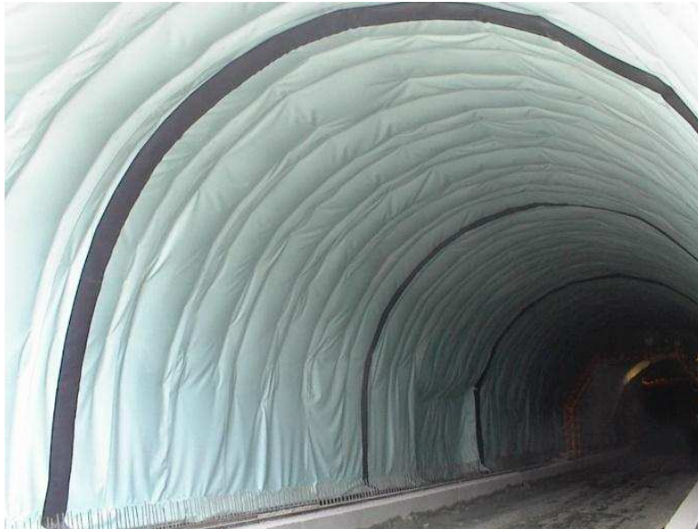
Fig 3. Waterproofing geomembrane system installed in a tunnel before casting of final lining
