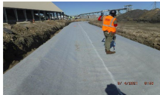
Fig. 4. View of the 1-mm thick GCL installed on the northern end of the West Ditch.
