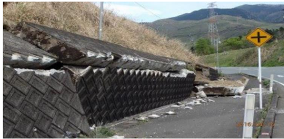
Fig. 1. Failure of retaining wall during the Kumamoto earthquake in Japan occurred on the 16th of April 2016 [2]
