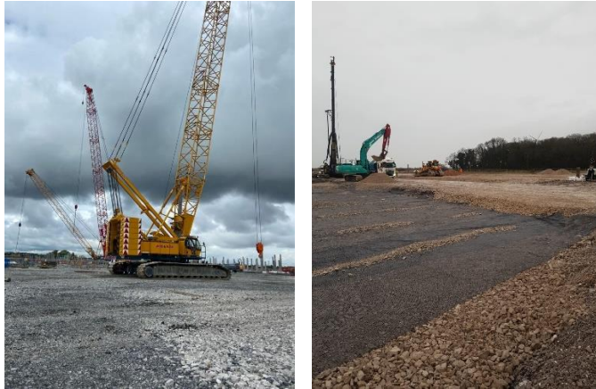
Fig. 7. The crawler crane and the construction of the working platform for Protos Efw project in UK
