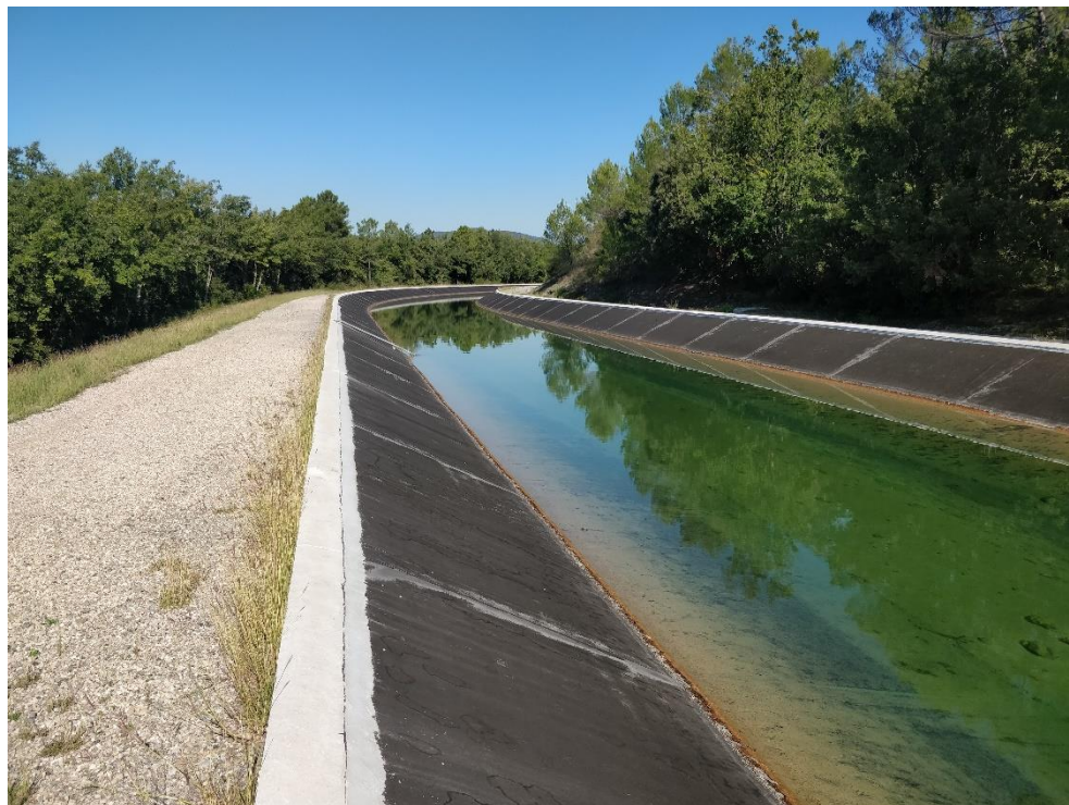
Fig. 1. BGM installed in Canal de Provence (France)
