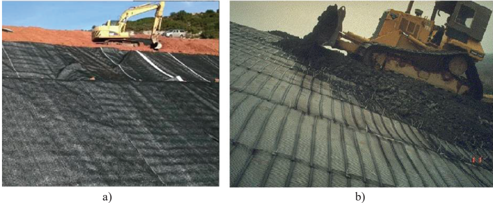
Fig. 4. Examples of soil veneer with (a) reinforced geomats and (b) uniaxial geogrids.
