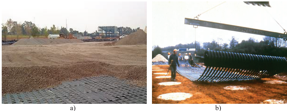
Fig. 3. Examples of basal reinforcement: (a) embankment on soft soil and (b) piled-based road embankment [8].
