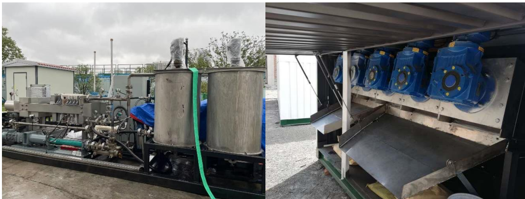
Figure 1. Stacked-screw machine (right) and plate and frame filter press (left).
