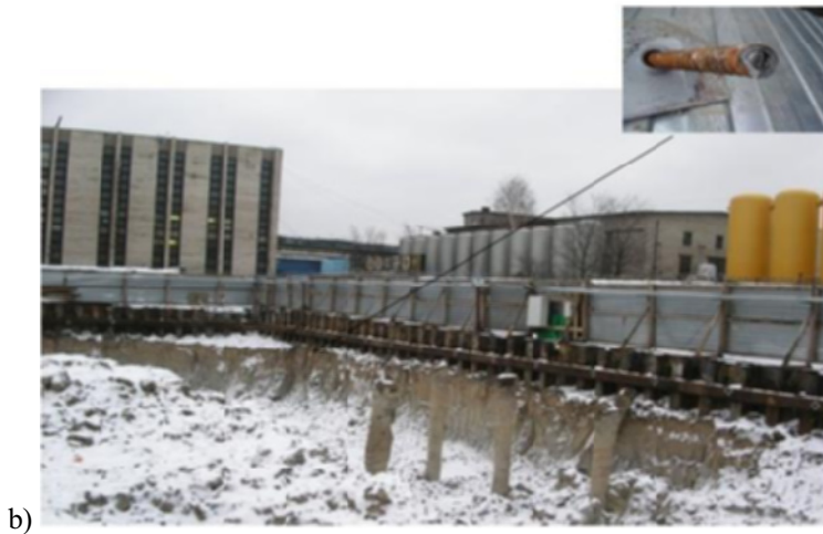
Fig. 1 a) Loss of stability of the pit struts; b) sheet piling anchor failure.
