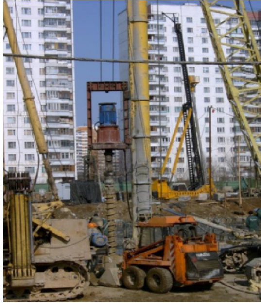
Fig. 3. The pile foundation installation process: 300 mm diameter RIT-piles in the foreground, Fundex piles in the background.
