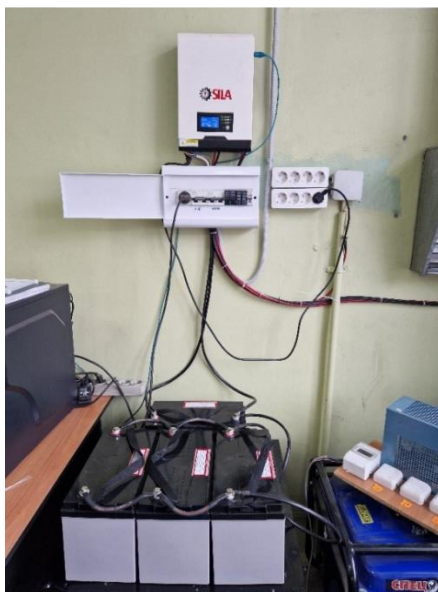
Fig. 3. External view of the battery pack with inverter.
