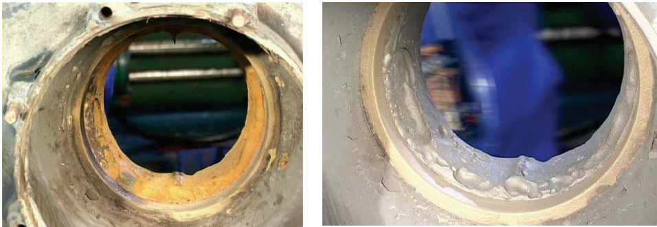
Fig. 2. Wear of pump volute internal surface.
