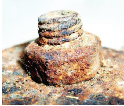
Fig. 3. Slots and corrosion products at the outer ends of fasteners.
