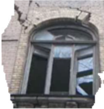
Fig. 1. Spatial kinematics of destruction in the form of vertical, horizontal and inclined cracks from dynamic impacts.
