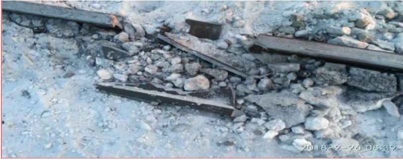
Fig. 2. Rail break at the derailment site.
