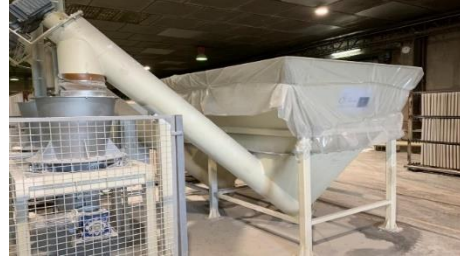
Fig. 3. Tank of shredded polyurethane
