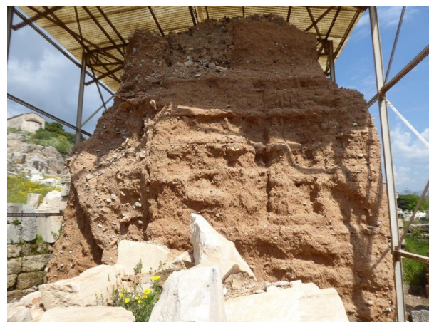
Fig. 1. Views of sections of the remaining volumes of mudbrick walls (photos taken 2020).
