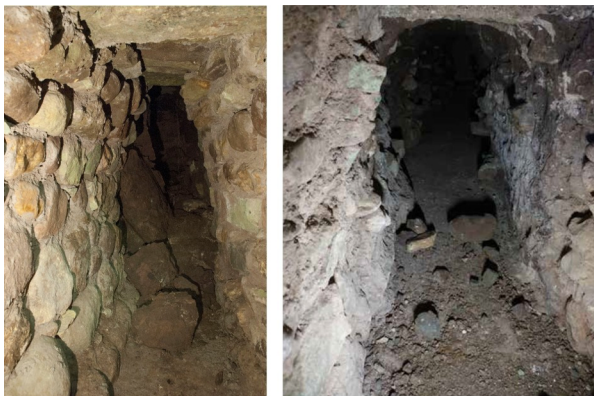
Fig. 5. Examples of local collapses at the interface between lined and unlined tunnels – left – and in an unlined tunnel – right [12].
