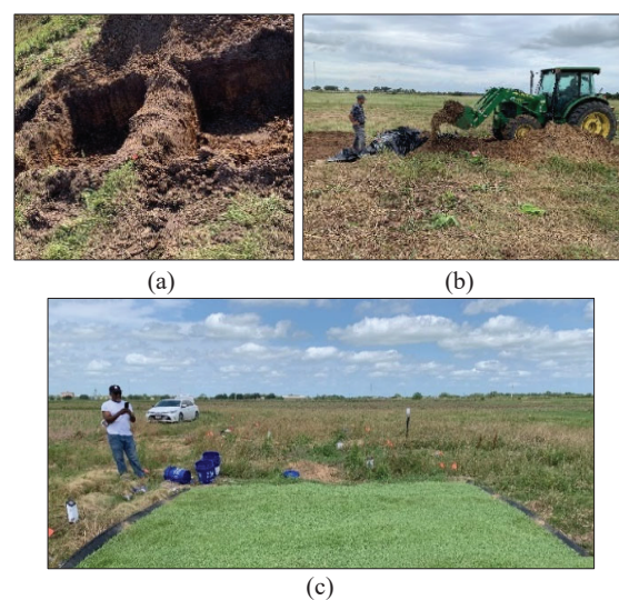
Fig. 1. (a) excavation of the test pits (b) soil backfilling after a 6-mil plastic sheet placed on the bottom of the excavation floor and inside the side wall of excavated pits (c) textured geomembrane layer placed over the smoothed compacted layer overlain by engineered turf
