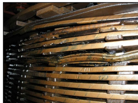
Fig. 11. Residual deformations of the HV winding of 250 MVA/500 kV/110 kV autotransformer with twisting of the winding and lodging of the turns on the edge.
