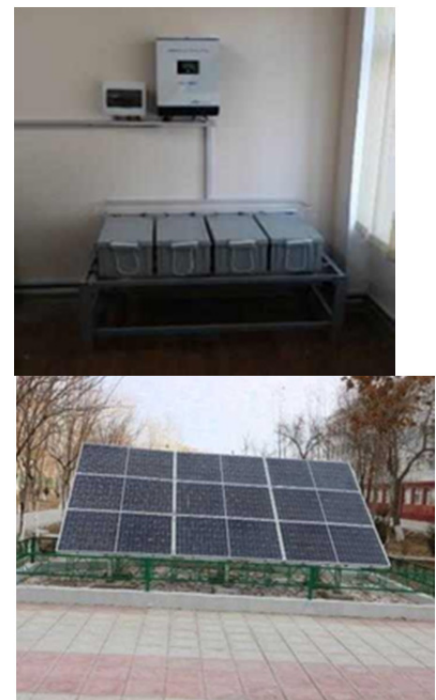
Fig.1. 3 kW photovoltaic system
