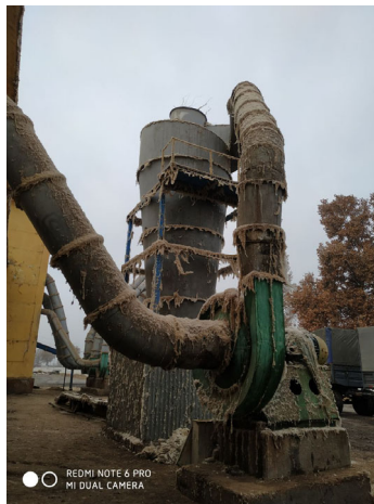
Fig. 4. The general view of the TS-6 cyclone separator in operation at ginnery.
