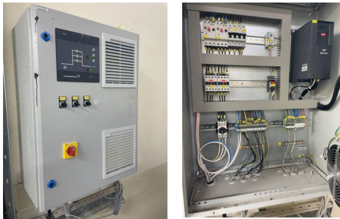
Fig. 1. General view of the pumping plant control cabinet.
