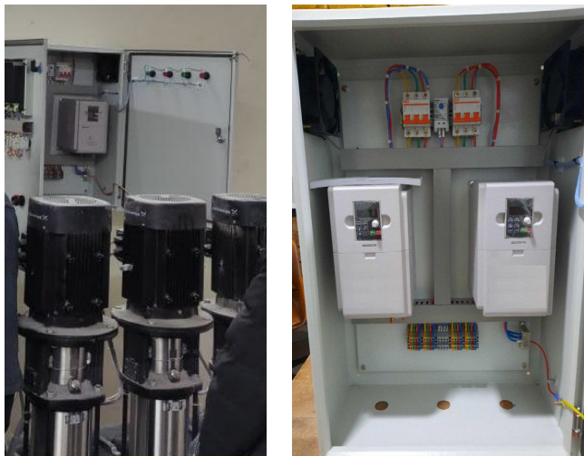
Fig. 3. General view of the energy efficient soft start device.
