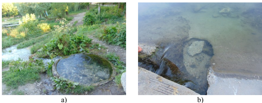
Fig. 2. Violations recorded on pond 21, located in the upper reaches of the Slavyanka river: a) erosion of the coastline; b) destruction of the bottom lining.
