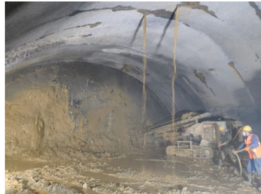
Figure 2: Tunnel lining water seepage
