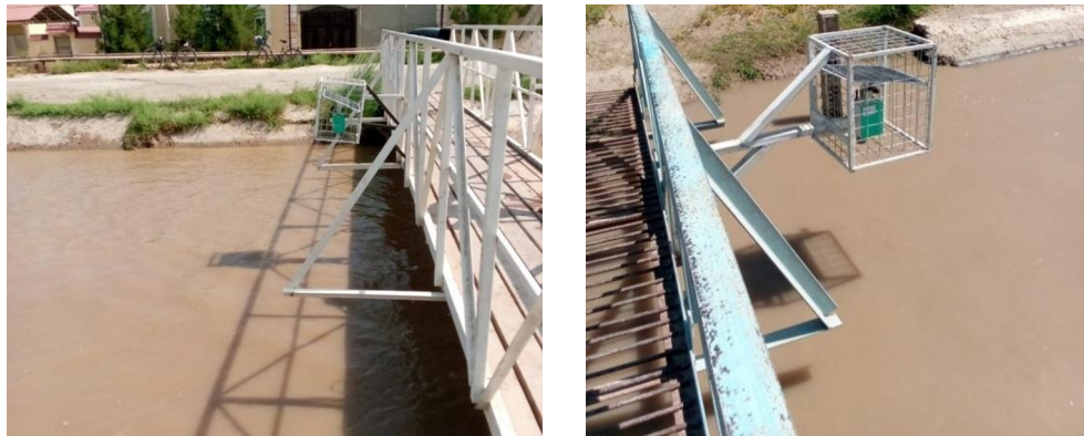
Fig. 11. Intelligent level sensors installed on the irrigation canals.
