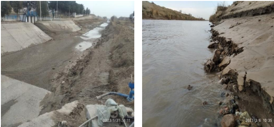
Fig. 2. Deformation processes in pickets PK 30-35 of Amu-Zang channel
