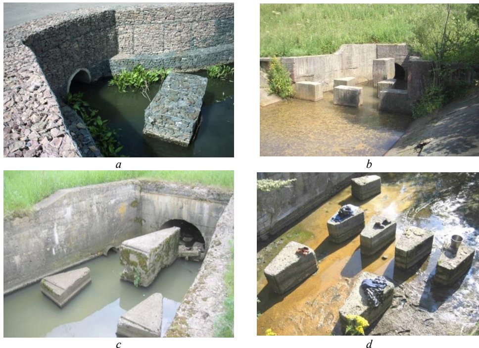
Fig. 1. Results of tubular culverts surveys held in Moscow Region, built according to standard designs of different years [3,5] (photo by the authors): a is deformation of fastening of downstream of single-point tubular crossing from corrugated pipe and gabion structures on Moscow-Kolomna highway, 2021; b is water well with dampers-spreaders behind two-point spillway of pond on river Chernichka in Podolsk region in 2009; c is fragments of building structures in pipe and at beginning of water well of dam on river Solovka, Podolsky district, 2019; d is displacement of absorber of second row of Ptitsegradsky pond on river Torgoshe, Sergiev Posad district, 2005.
