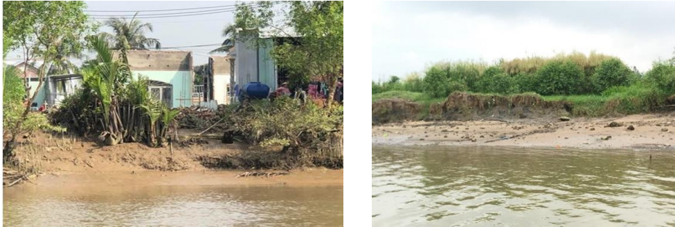
Fig. 1. Erosion on bank of Sai Gon River
