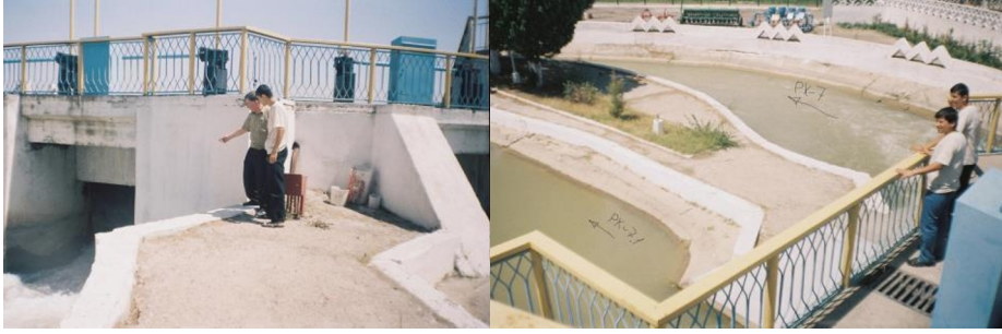
Fig. 1. The main hydraulic structure of the rk-7 channel
