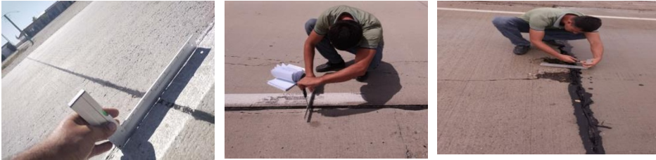
Fig. 4. Photographs of the change in the width of the grooves of the transverse expansion joints in section 315-320 km of the A 380 highway (2022).
