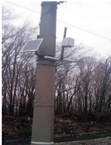
Fig. 5. Base station with antenna and solar battery
