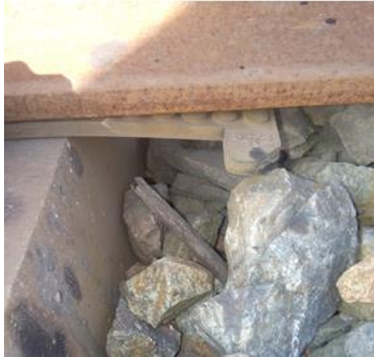
Fig. 2. Displacement of the under-rail linings along the sleepers.
