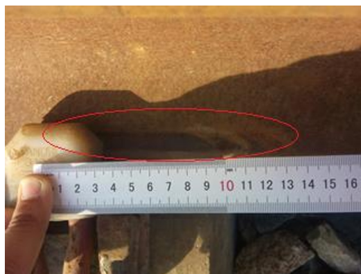
Fig. 1. Traces of the terminal on the sole of the rail at the longitudinal displacement of the lashes.
